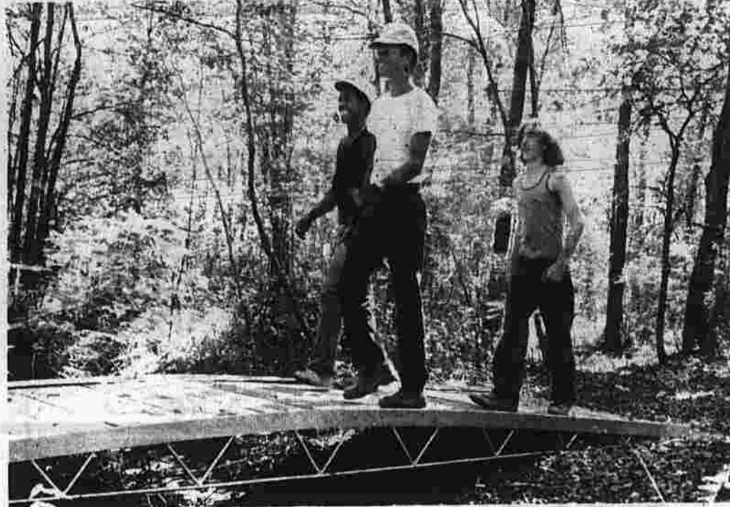
Jake Matthews (left), Mike Mack and Anthony Debonee (right) walk across a foot bridge they constructed with the help of six other workers. The bridge is part of a 2.5-mile nature trail and cross country ski course. The trail is located on 41.7 acres of wooded property just north of the East Hartford Golf Course. (Herald photo by Blake)
